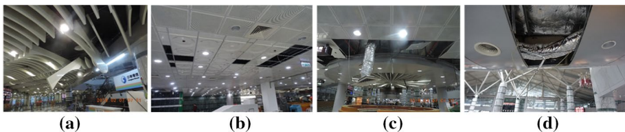
Fig. 19 a Fallen baffle boards, b fallen metal ceilings, c a ventilation duct hanging through the hole where the ceilings fell, and d a damaged sprinkler pipe used for fire-fighting in an airport terminal
