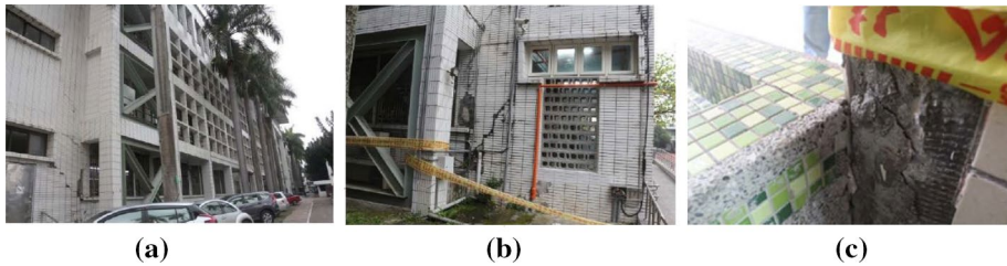
Fig. 16 a and b Cracked brick walls. c A cracked column of a four-story school building
