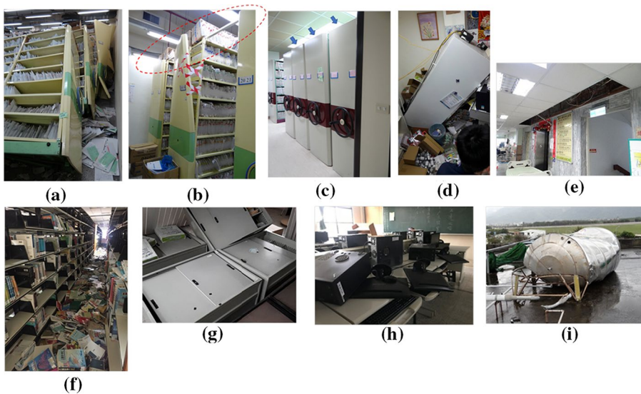
Fig. 18 a–c Damaged shelves for medical history sheets in a hospital. d An overturned medicine refrigerator. e Fallen ceilings in a hospital. f Books fallen from bookshelves. Overturned g filing cabinets and h desk computers. i A damaged water storage tank
